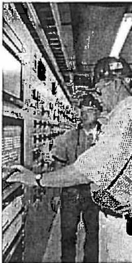
Views of the upgraded and expanded Ward Hill sub-station in Haverhill, Mass.
